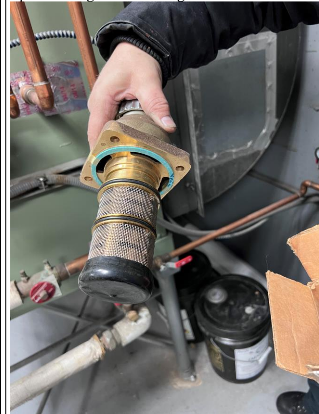
Spare mixing valve cartridge
